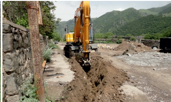
Hayastan All Armenian Fund – Argentina branch funded the construction of the water supply system in the occupied town of Kalbajar | Photo from www.himnadram.org | August 2013
