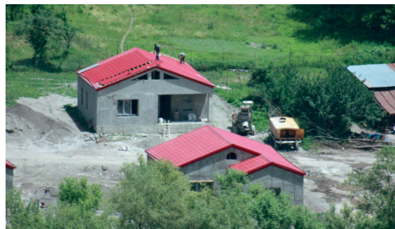
Construction of a newly housing in the occupied Lachyn district, funded by “ARI” Company | Photo from www.arirroots.com
