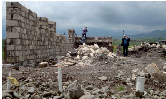
Hayastan All-Armenian Fund's Toronto (Canada) affiliate sponsors construction of a community centre in the occupied town of Khojaly | Photo from www.himnadram.org | 15 May 2015
