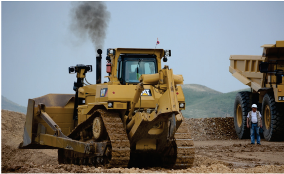
Caterpillar heavy machines are used in the exploitation of Demirli copper-molybdenum mine | Photo from www.bm.vallexgroup.am | 27 May 2014
