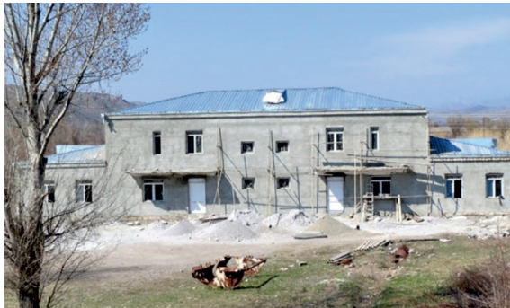
Construction of a ten-apartment building for the Syrian Armenian settlers in Khanlyg village of the occupied Gubadly district | Photo by Alvard Grigoryan | www.kavkaz-uzel.ru | 25 March 2014
