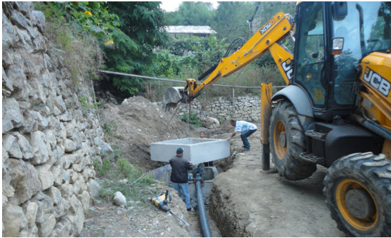
Construction of water supply system in the occupied Shusha district | Photo from www.himnadram.org | 2013
