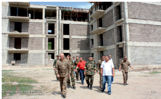
Construction of a new residential building in the occupied town of Kalbajar | Photo from www.president.nkr.am
