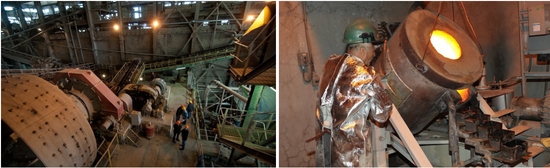
Ore from Soyudlu gold mine is processed at Ararat Gold Processing Plant in Armenia | Photo from www.geopromining.com
