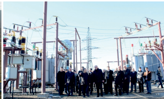
Newly built transformer substation in the vicinities of the occupied town of Shusha | Photo from www.president.nkr.am
