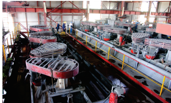
Ore processing plant at the Gyzybulag underground mine near Heyvaly village in the occupied Kalbajar district | Photo from www.bm-old.vallexgroup.am
