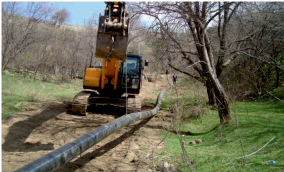
Second phase of the construction of the water supply system in the occupied town of Lachyn | Photo from www.himnadram.org | April 2013
