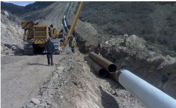
Armenia’s Dorozhnik LLC company built transmission pipeline for water flow of Toraghaychay River in the occupied Kalbajar district into the Sarsang reservoir
