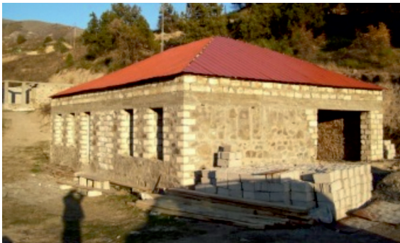
New house for a Syrian Armenian family is built in the occupied town of Lachyn | Photo from www.friendsofarmenia.com | 02 September 2013
