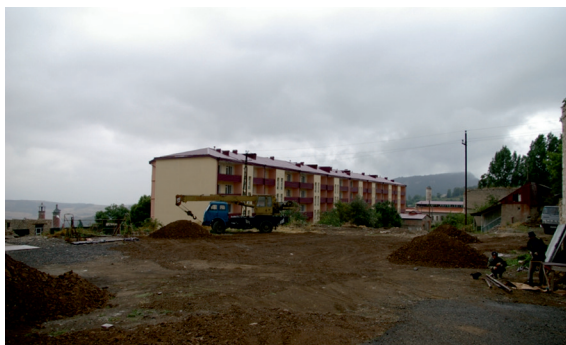
Construction/Reconstruction of a residential building in the occupied town of Shusha | Photo by Christian Garbis | www.noteshairenik.blogspot.com 07 August 2011
