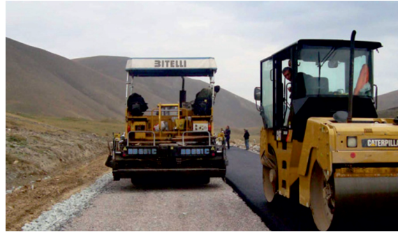
Construction works at the Vardenis-Aghdara highway passing through the occupied Kalbajar district of Azerbaijan | Photo from www.armenianfundusa.org | 10 November 2014
