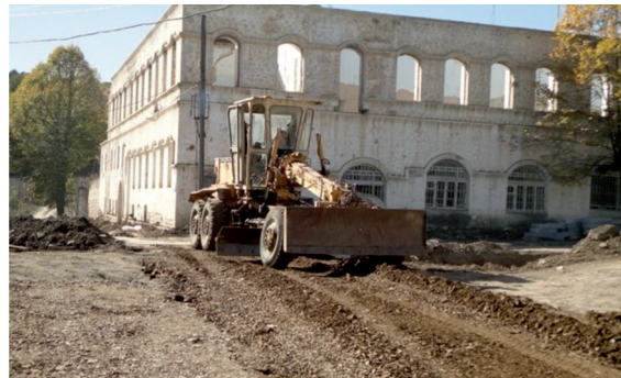
Hayastan All-Armenian Fund funded the reconstruction of the road infrastructure in the occupied town of Shusha | Photo from www.himnadram.org | August 2011
