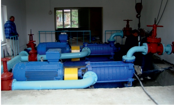
Hayastan All Armenian Fund funded the reconstruction of the water supply system in the occupied town of Lachyn | Photo from www.himnadram.org | June 2011
